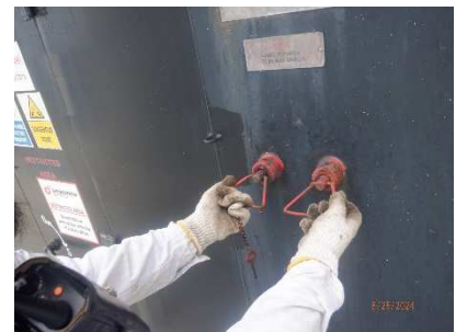
9) shutting off Damper
