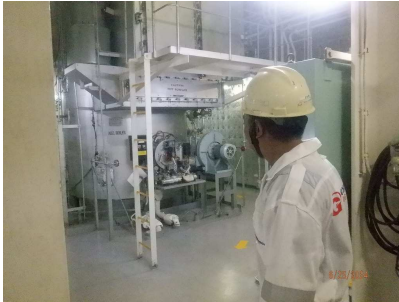
1) Duty engineer detects the fire
